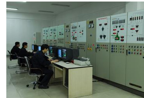
Rubber mixing microcomputer monitoring room
