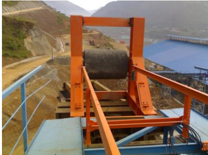
Discharge Pulley Station
