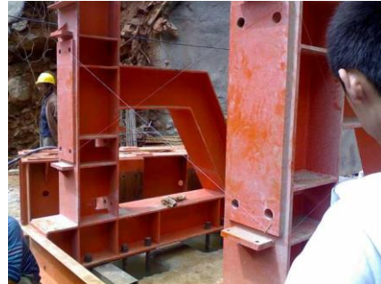
Tail Pulley Station
